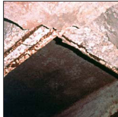
Spalled concrete beams
