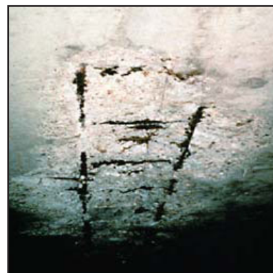
Deteriorated overhead concrete
