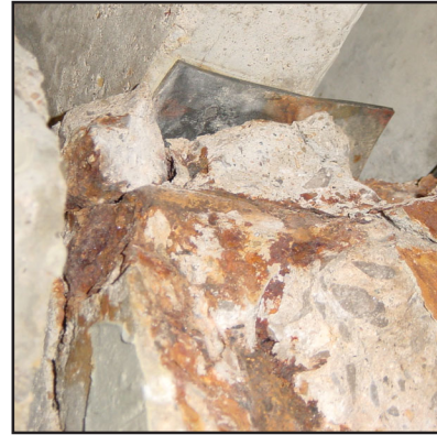
Corroded steel and concrete deterioration at a column and beam connection
